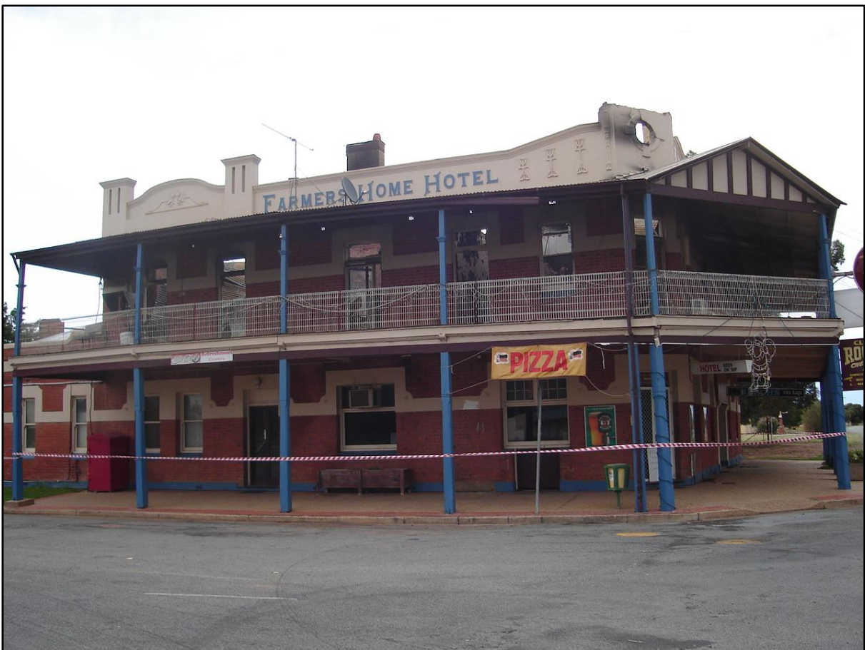
Above and Below: The Farmer's Home hotel in February 2008, after the fire had gutted the building.
