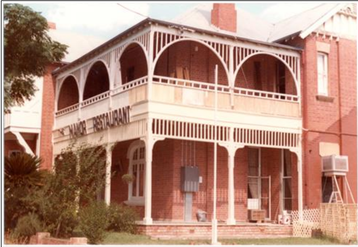
Above: A photo showing the restoration of the verandah openings back to their original status – the added windows and partitions that were installed to create additional rooms have been removed. Courtesy James Little.
