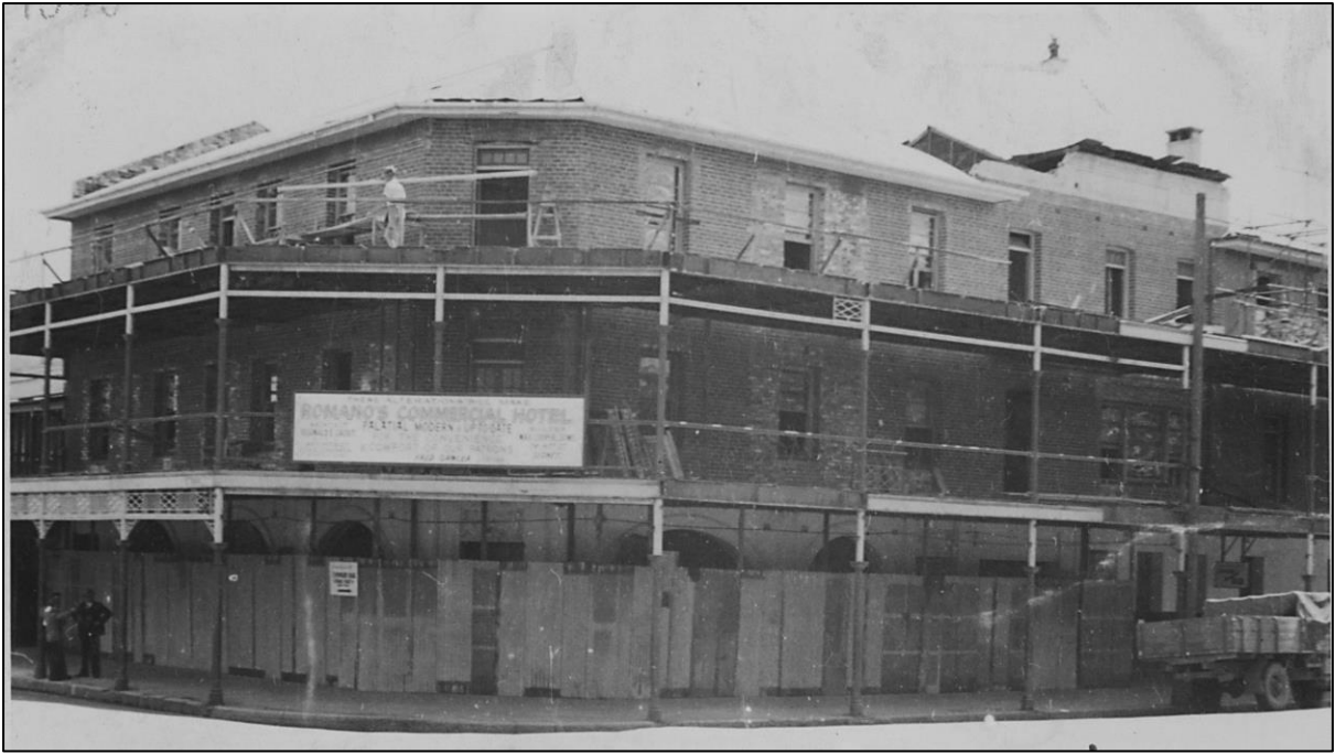
Above: Stripping the external façades back ready to remodel the hotel in 1949. Courtesy Tooth & Co.
