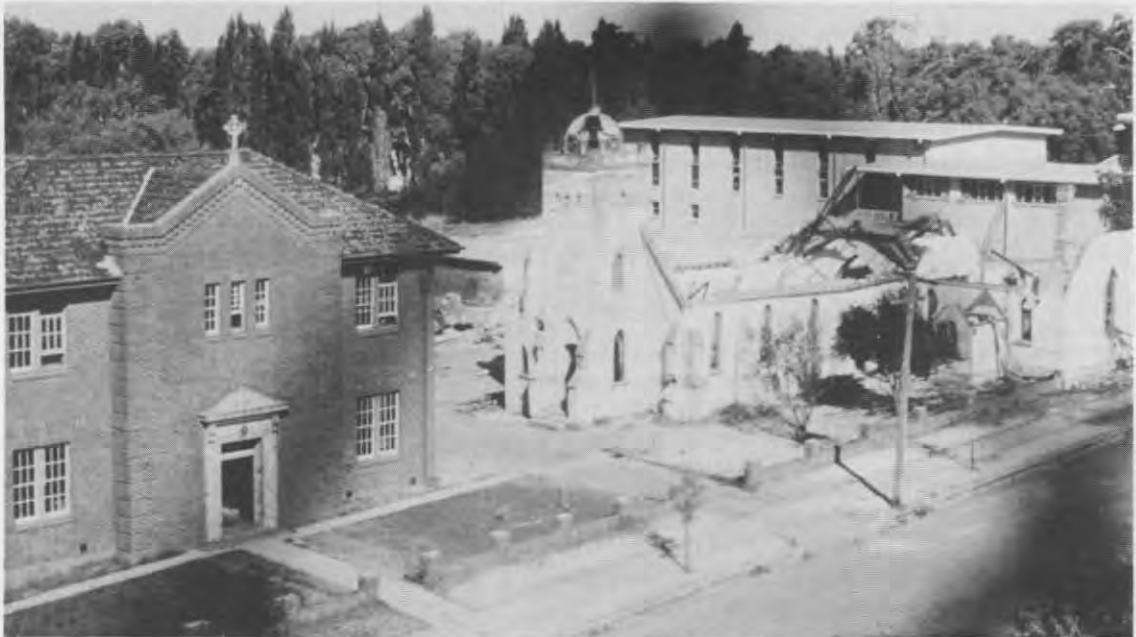
Demolition of first Saint Michael's Church and School in 1965 Christian Brothers' High School in foreground
