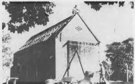
Stable in which the Sisters taught in 1874, in process of demolition in 1959
