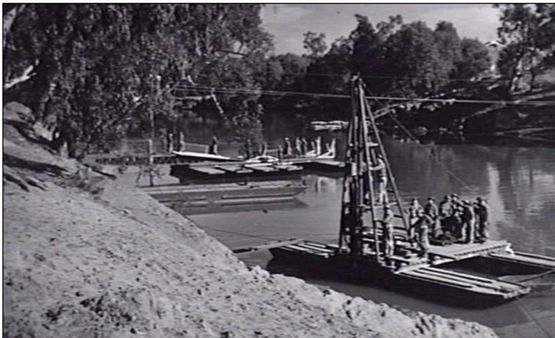
Above: Using a pile driver to construct a jetty at Wagga Wagga. Courtesy Australian War Memorial. [052556].
