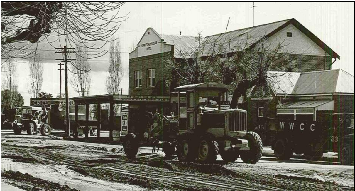
Above: Roadworks in front of the hotel. The top part of the verandah has been removed, but not the bottom part.
