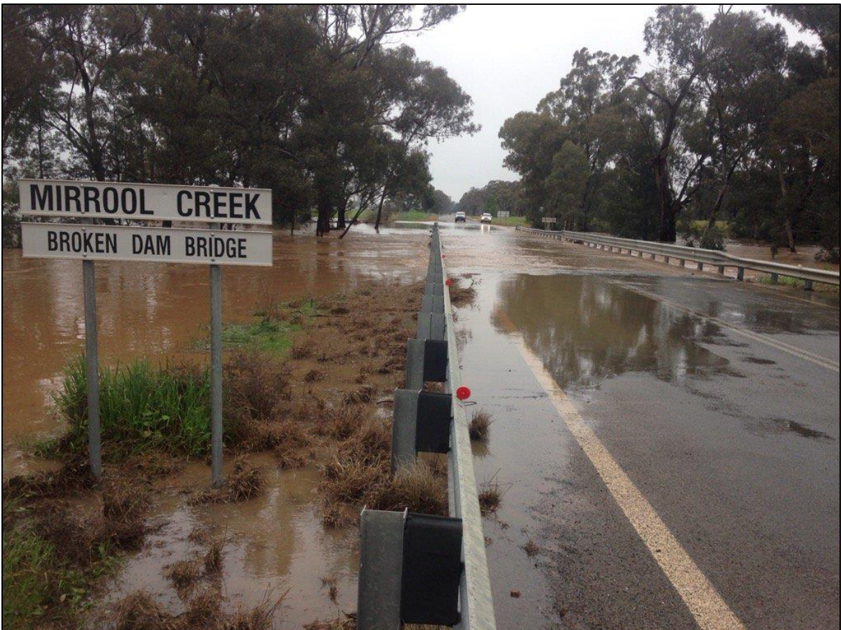
Above: A view of the contemporary bridge during a major flood in 2016. Courtesy Darryl Harper.
