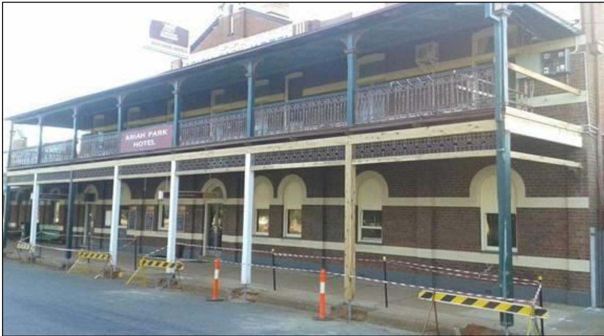
Above: 2016 works on the verandah and the footpath. Courtesy Ariah Park Hotel Facebook page.
